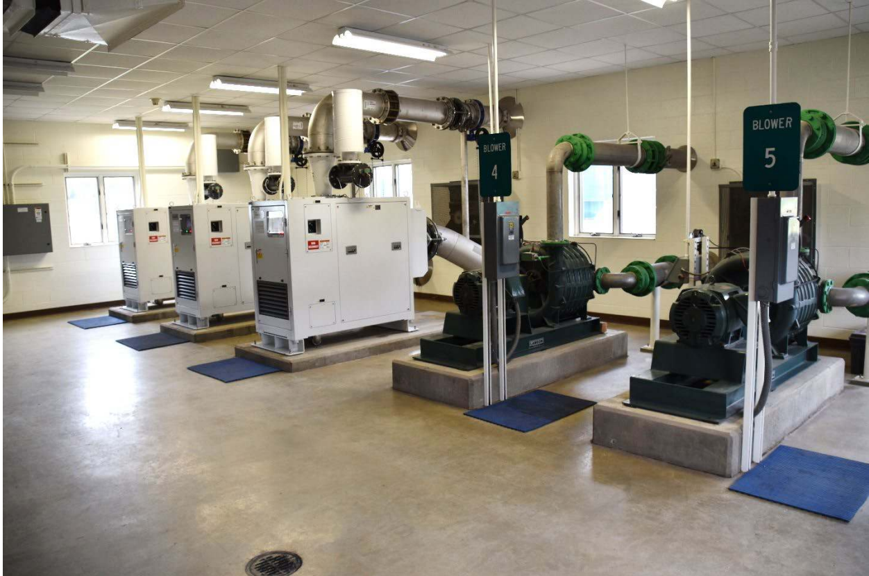
Picture showing turbo blowers next to old centrifugal blowers.
