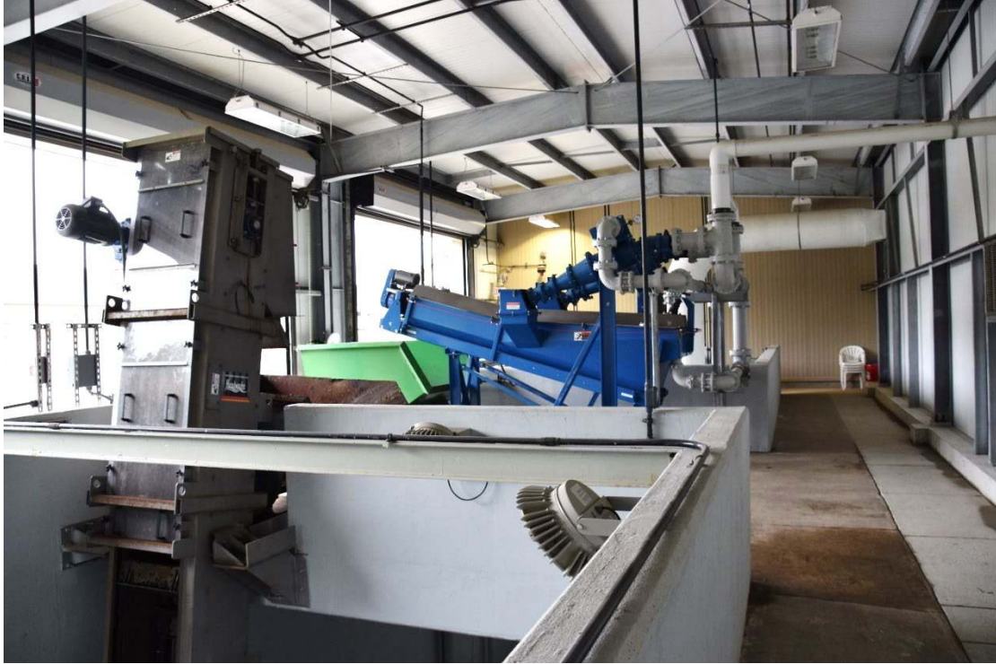
Picture of Plymouth's below ground headworks.
