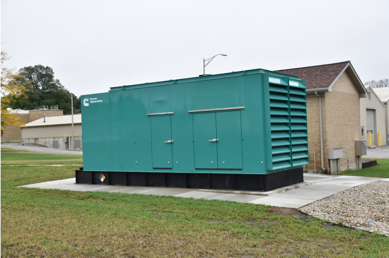
Example Stand By Generator
