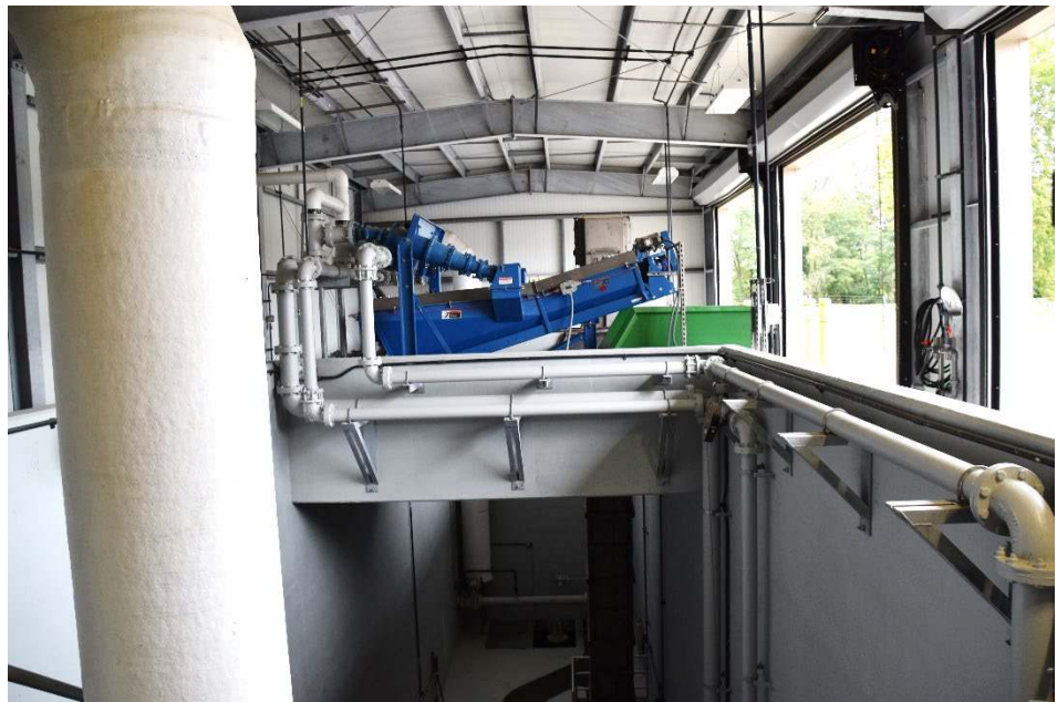
Picture of Plymouth's below ground headworks.
